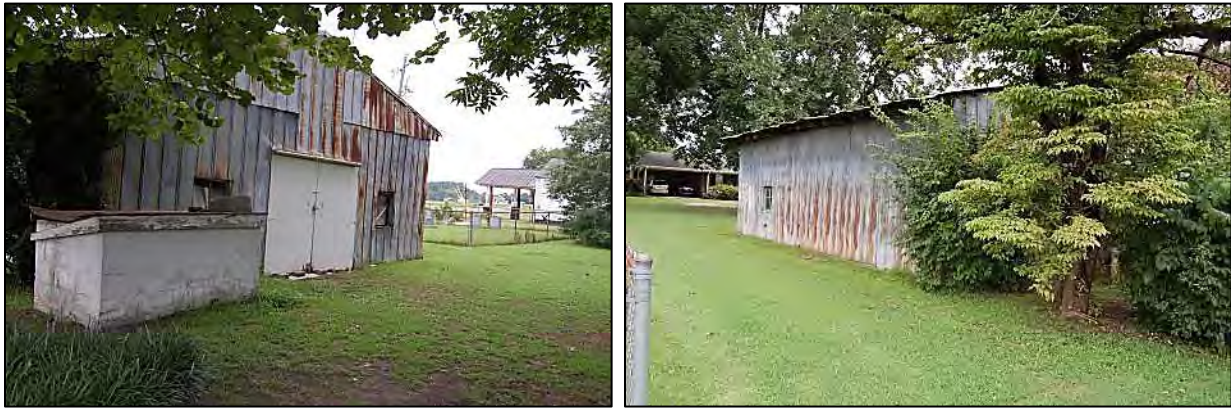
Figure 135: Shop: to left, south rear elevation with cemetery and Stroud Store beyond; to right, east side and north front (in trees) elevations, with Billy Baker House to rear.
