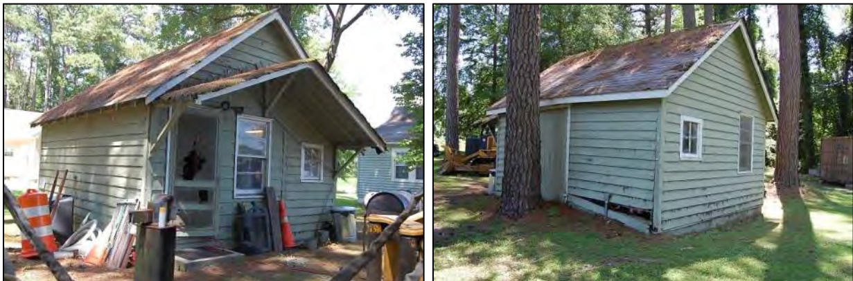
Figure 299: Kelly's Pond Lookout Tower: west side and south front elevations of workshop, at left, and east side and north rear elevations, at right.
