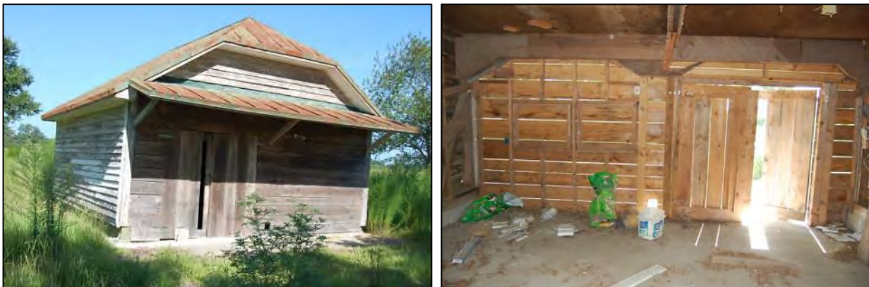
Figure 78: South side and east front elevations of garage, at left, and interior view showing alterations, at right.
