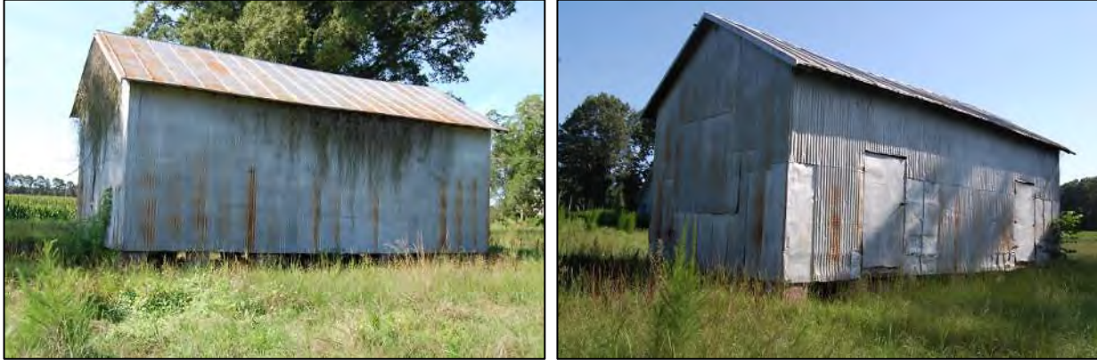
Figure 81: At left, west elevation of packhouse, at right, south and east elevations.
