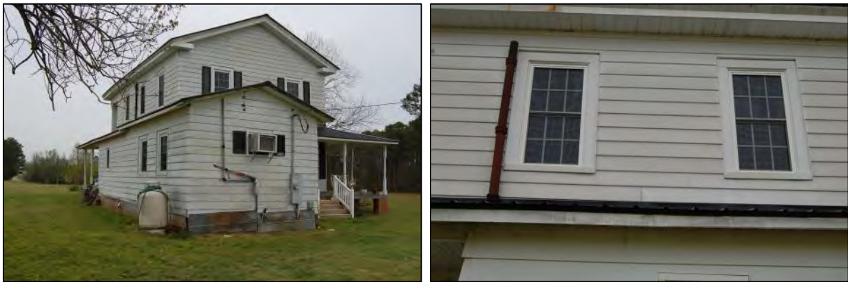
Figure 287: Wooten-Whaley House: west rear and north side elevations, at left; second story of north side elevation, at right.
