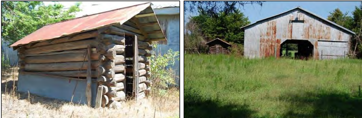
Figure 234: At left, south side and east front elevations of log crib; at right, east-facing gabled elevation of barn.
