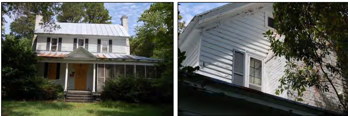
Figure 12: Tull-Worth-Holland House: south front elevation and east side elevation detail depicting intact boxed cornice, beaded weatherboards, and surround, 2017.
