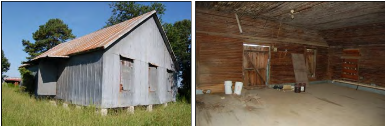
Figure 82: Left, view of northeast corner of Shed, looking southwest; right, view of interior of shed, looking south.
