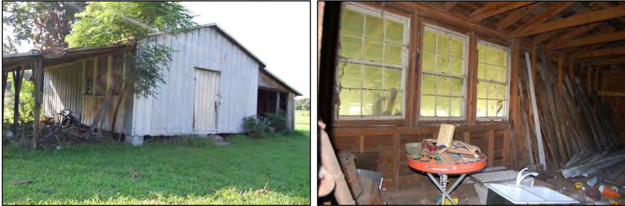
Figure 266: Left, view of western elevation of striphouse; (looking east); right, interior view of striphouse windows.
