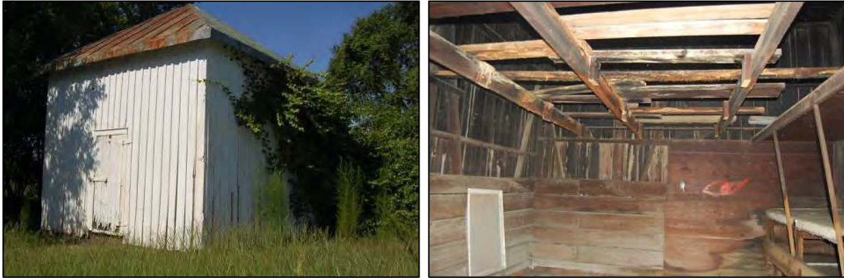
Figure 79: View looking northeast at smokehouse, at left, and smoke-stained interior, at right.
