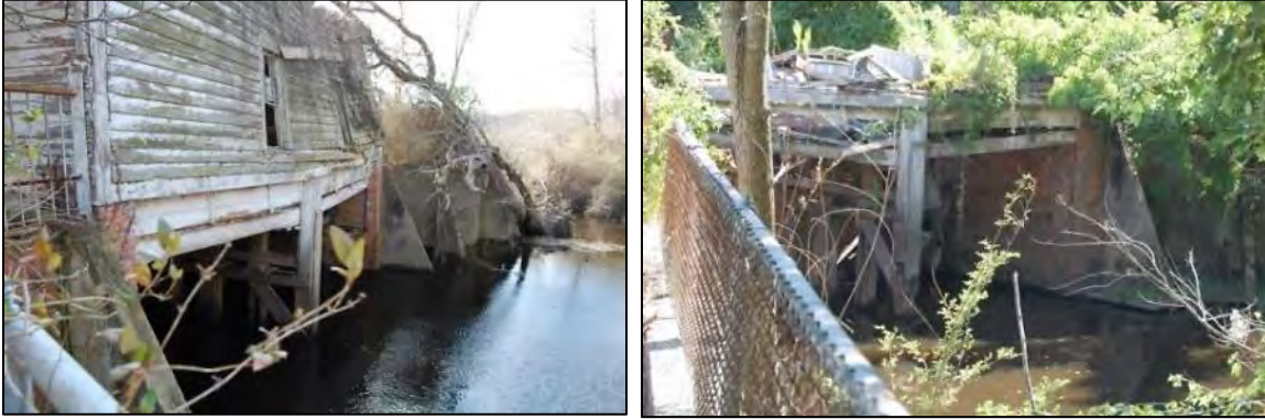
Figure 252: At left, view of north elevation of Kelly's Mill, 2010; at right, same view, 2017.
