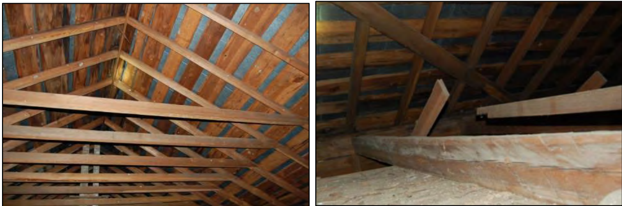
Figure 171: Croom Meeting House: at left, view of replacement roof trusses; at right, original roof tie beam that appears to be pit-sawn.
