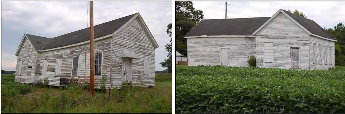
Figure 113: Tyndall School: at left, looking northeast with front block at right; at right, looking northwest with rear block at right.
